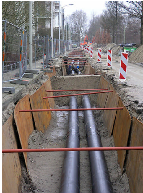
An example of DH pipes used in a CHP system
